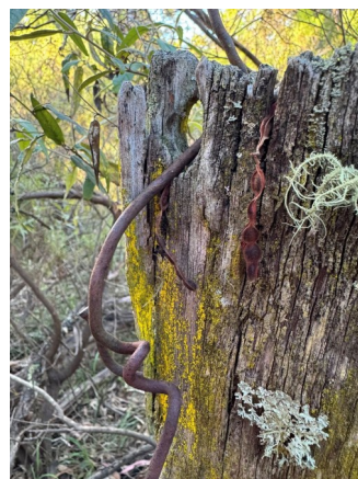
Poignant reminders of failed attempts to tame the forest.
